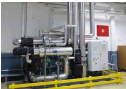
Oil/hot water heat exchanger
