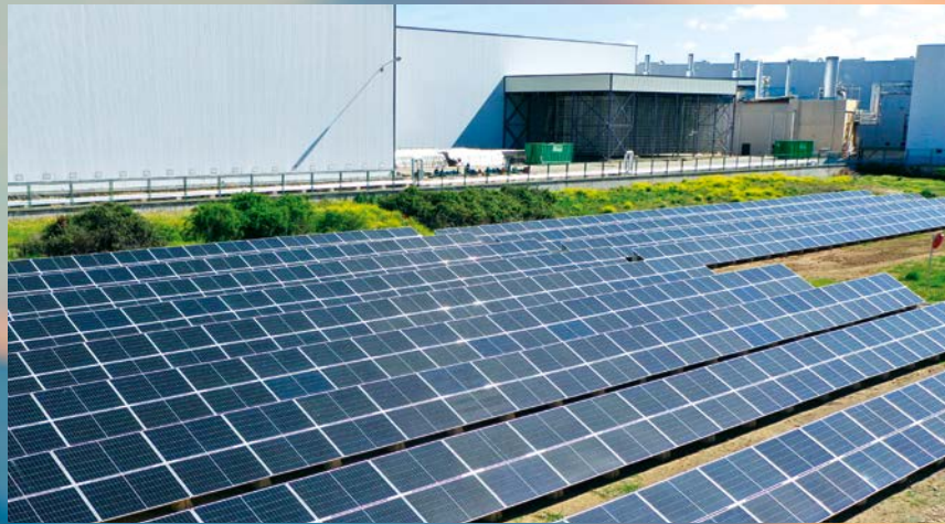
The energy generated by the solar system will be > 500,000 KWh/year
