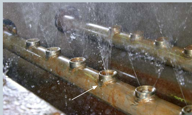
Fig. 4: Uneven water application due to disturbed fan jet
