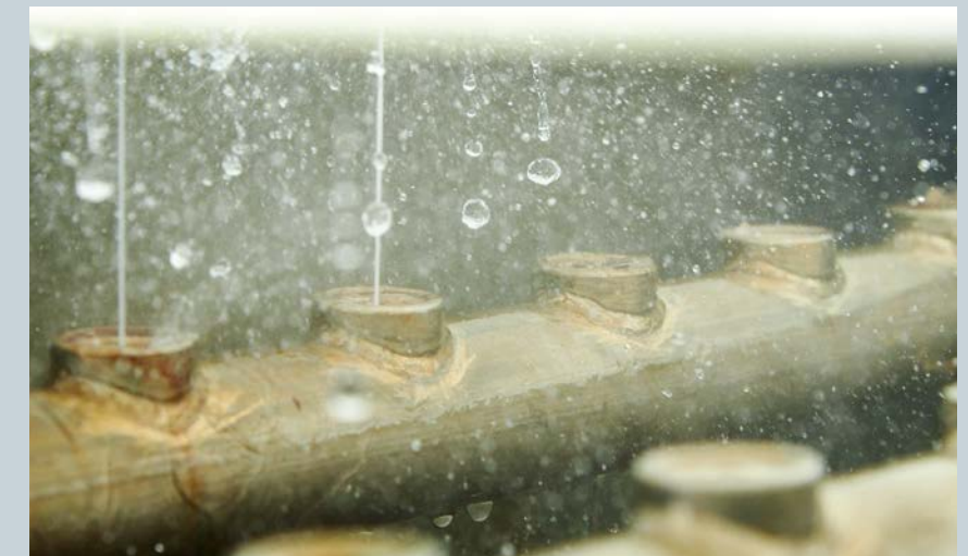
Fig. 2: Functioning and clogged nozzles
