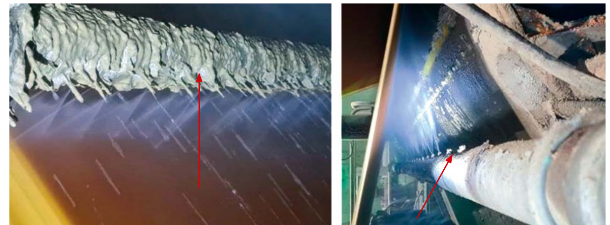
Fig. 4: shower pipes showing dirt deposits and partially clogged nozzles
