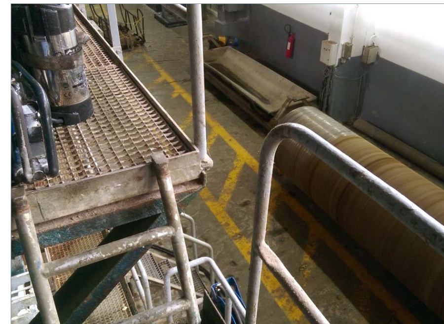
Risk of falling
