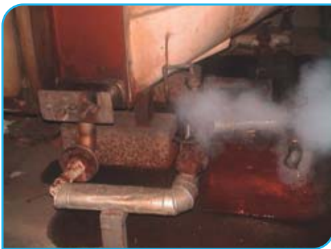
III.6 Leaking pipework
