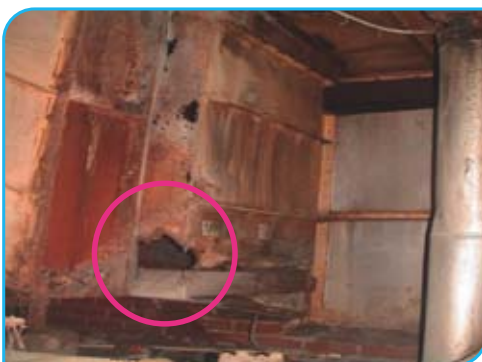
III.7 Corrosion on heat exchanger
